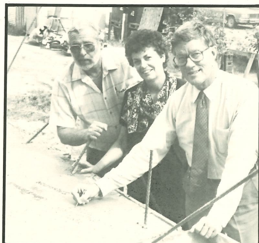
Contractor Jerry Albritton, Assistant to the Dean JoAnn Blackwell and Dean Sandy D'Alemberte record their signatures in the concrete foundation of the rotunda addition.
