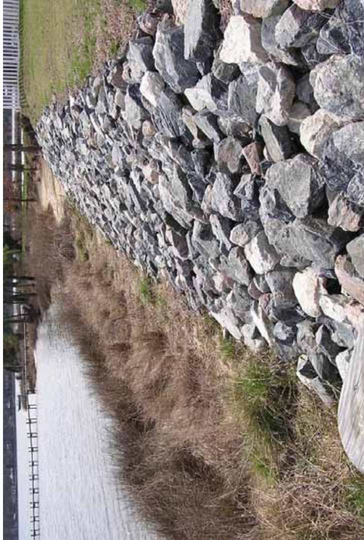
Conventional Revetment Reproduced courtesy of the Center for Coastal Resource Management, Virginia Institute of Marine Sciences
